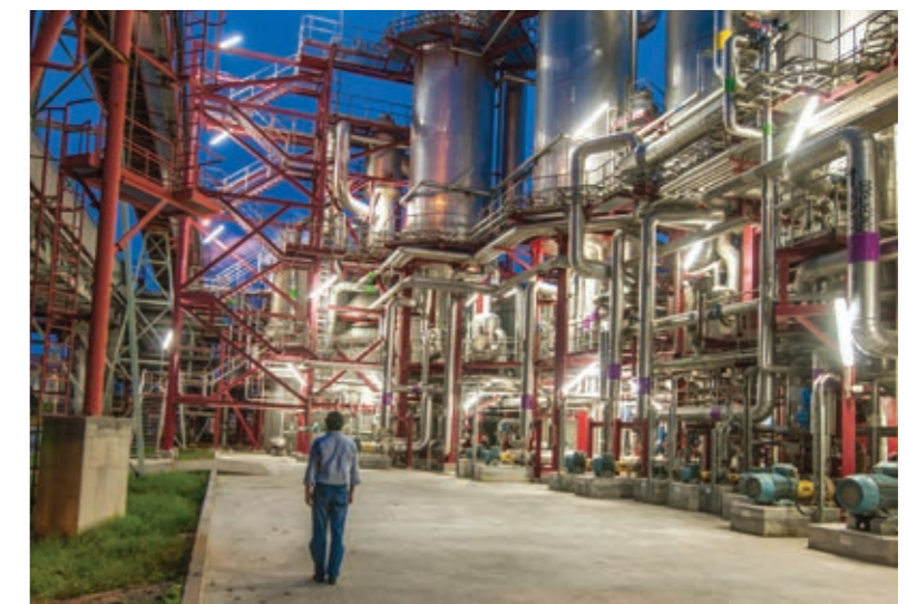
The new Navigator biomass boiler at Figueira da Foz is an important step on the road to carbon neutrality at the Company's industrial complexes.
